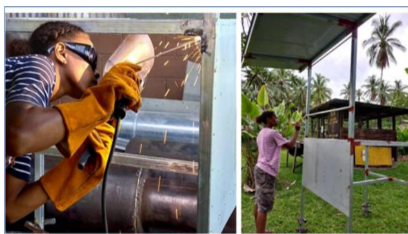
Figure 23. Fabrication and installation of water sink basins at PNG Agriculture Company buying points in East New Britain.
