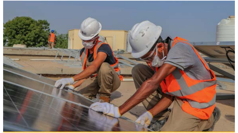
Workers install solar panels to power a public hospital in Yemen, restoring operations affected by ongoing conflict.
